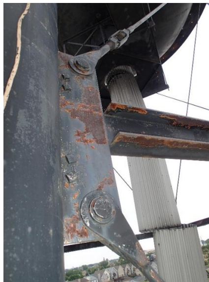
Figure 6: Corrosion at steel connection plates
