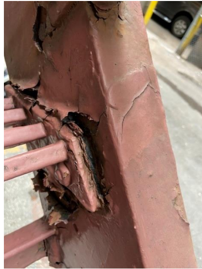
Figure 4: Corrosion built up between fire escape steel stringer and stair tread
