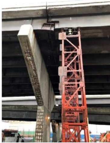
Figure 7: Cracked steel girder
