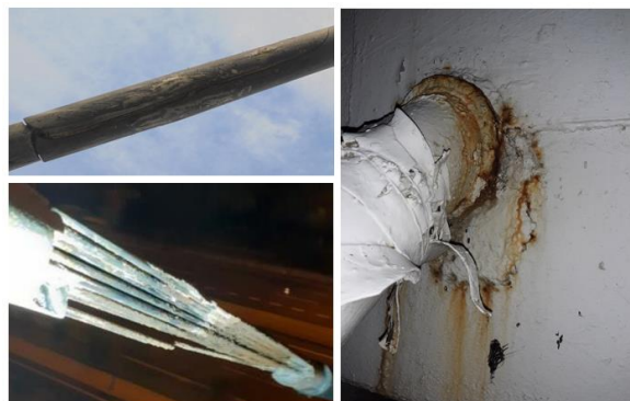
Figure 4: PWS cable recorded during inspection stage
