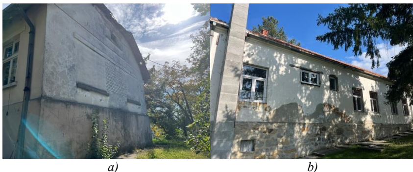
Figure 6: General appearance and damages of a school building a) in village of Arapovac, and b) in village of Mirosaljci
