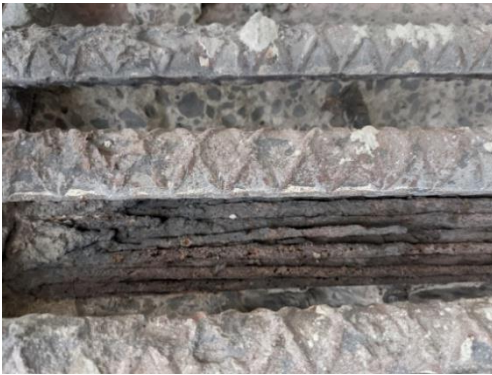
Figure 3: Fractured and heavily corroded girder tendon exposed in a concrete repair opening
