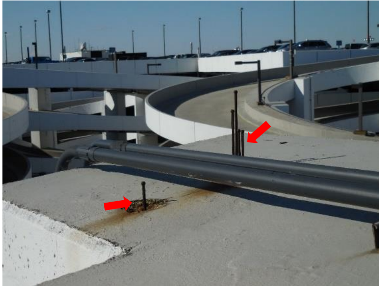
Figure 10: Failed post-tensioning wires erupted from top of a helical ramp column
