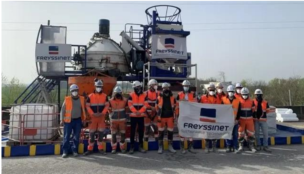
Figure 2: UHPFRC Batching plant (source Freyssinet)
