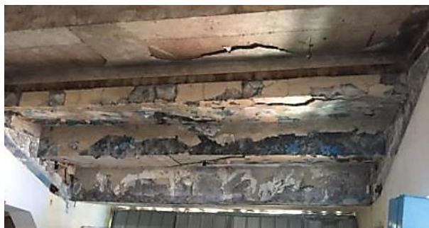
Figure 5: Damage to the reinforced concrete grandstand structure
