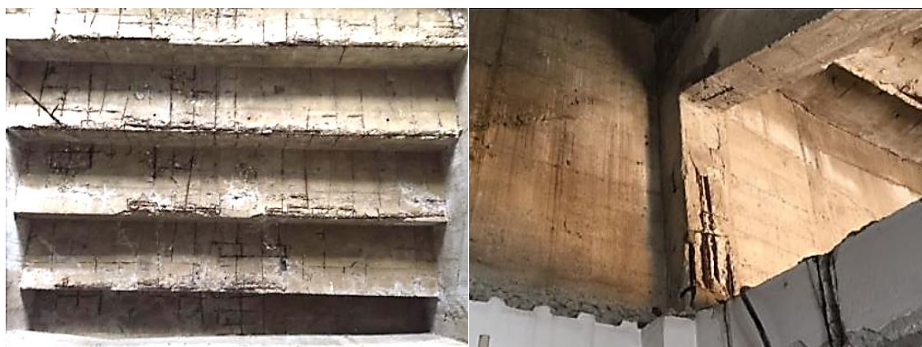
Figures 3 and 4: Damages to the reinforced concrete grandstand structure
