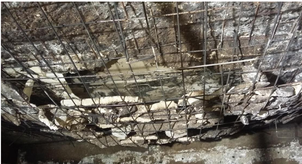
Figure 4: Complete degradation of the concrete and collapse of the RC floor slab between Axes 2 and 3
