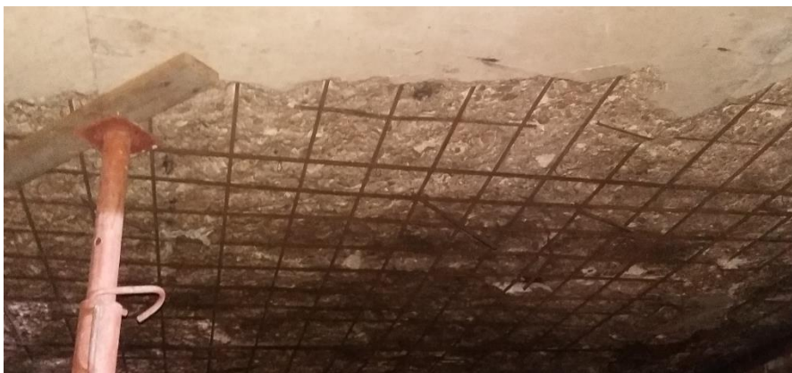
Figure 5: Extensive spalling of the concrete cover of the RC floor slab between Axes 1 and 2
