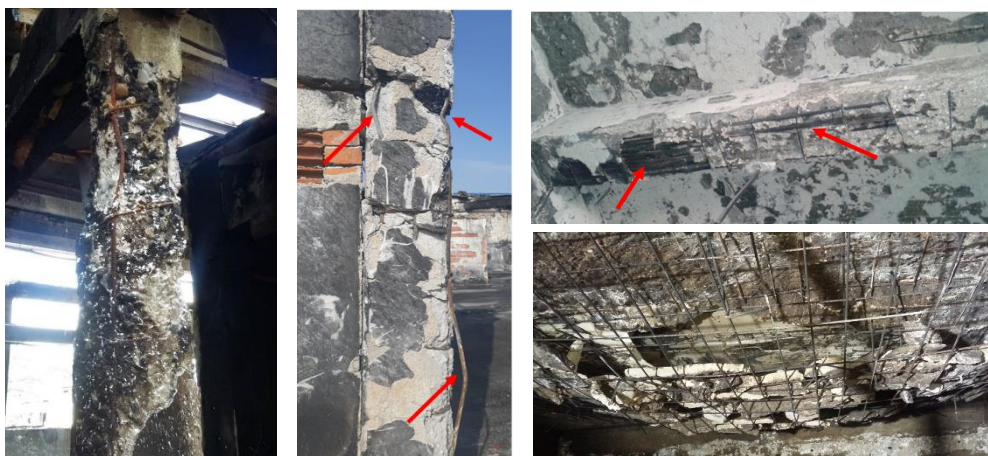
Figure 1: Examples of fire-damaged RC structural elements
