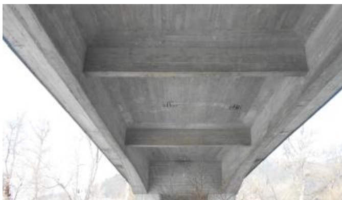
Figure 2: Present state of the girders
