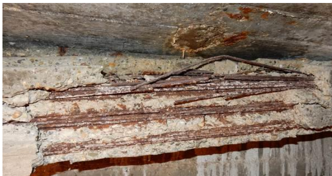
Figure 3: Broken wires in the upper row of the prestressing tendon on axis B, damp stains and traces of rust around the openings used for the subsequent concreting of the tendon
