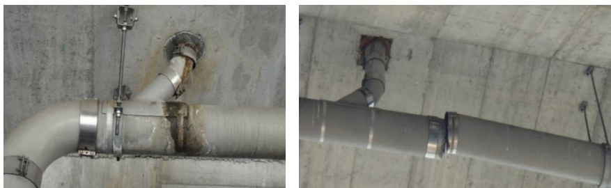
Figure 7: Unsatisfactory condition of drainage system components on the underside of the Ada Ciganlija Bridge structure
