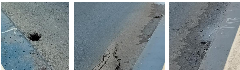
Figure 2: Drainage openings in the structure of the Branko's bridge and pavement deformations prevent effective drainage even during relatively moderate rainfall events
