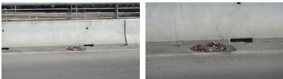
Figure 6: Unmaintained drainage inlets on the Ada Ciganlija bridge
