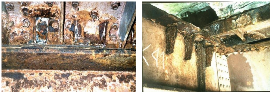
Figure 4: Condition of the Gazela Bridge structure resulting from corrosion of the steel box girders prior to the 2012 rehabilitation
